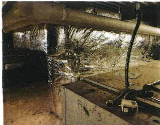
Mixed Air Duct
