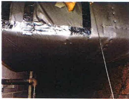
Supply Air Duct in Ceiling Plenum
