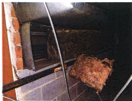
Return Air Opening (Blocked Off)
