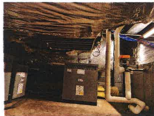
Return Air Damper in Mech. Room.
